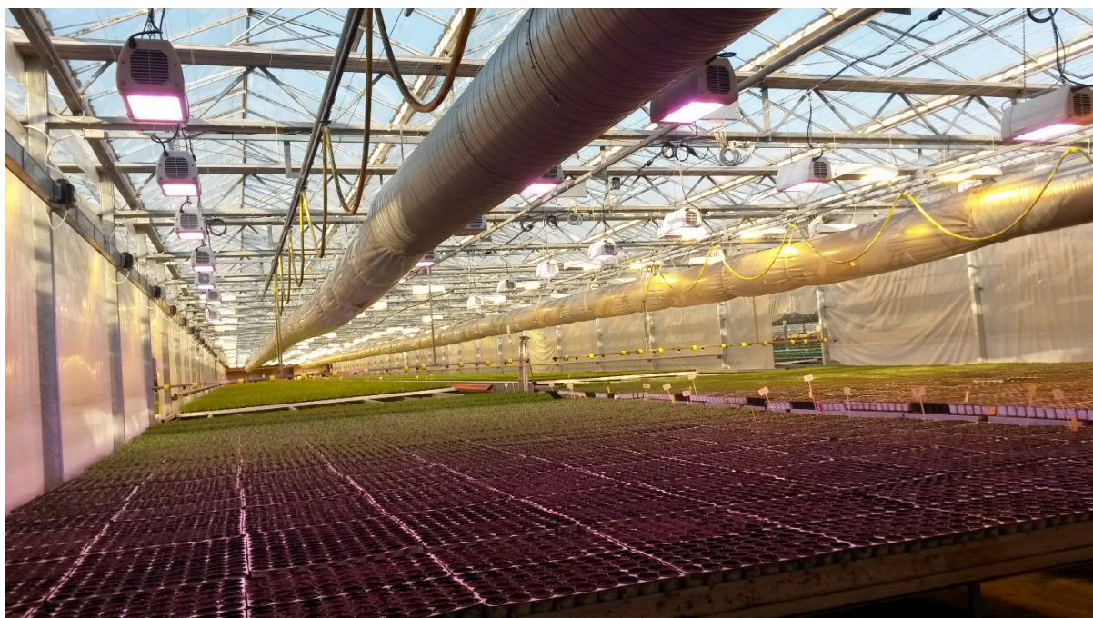
Picture: Heliospectra LX60 installed in greenhouse at Swedeponic
